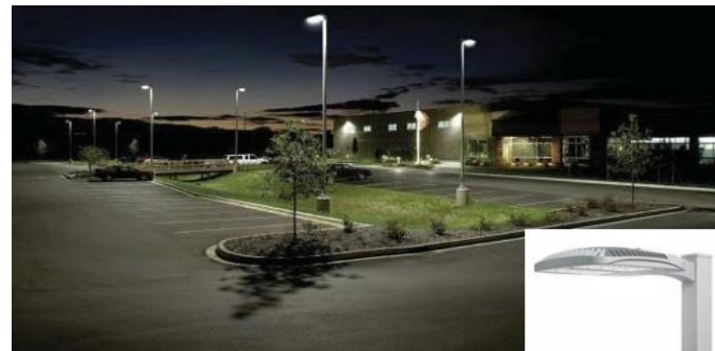
Parking Lot Lighting
